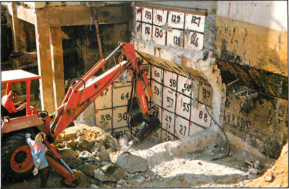
Figure 5. Standard or slightly modified demolition techniques can be used for many decommissioning operations. (Photo: Rockwell International)
